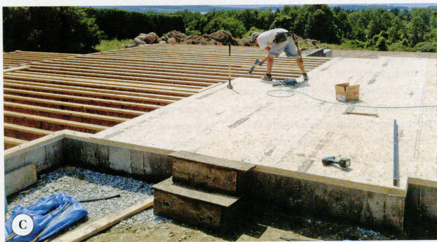
Figure 3. The LVL beams that support the first-floor framing are included in the JobPack package, along with supporting columns, metal connectors, and even the dimensional lumber used to frame the supporting walls (A). Joist layout is premarked on the LVL beams and LSL rim joists (B), which streamlines joist installation and allows the crew to quickly get the deck sheathed (C).
